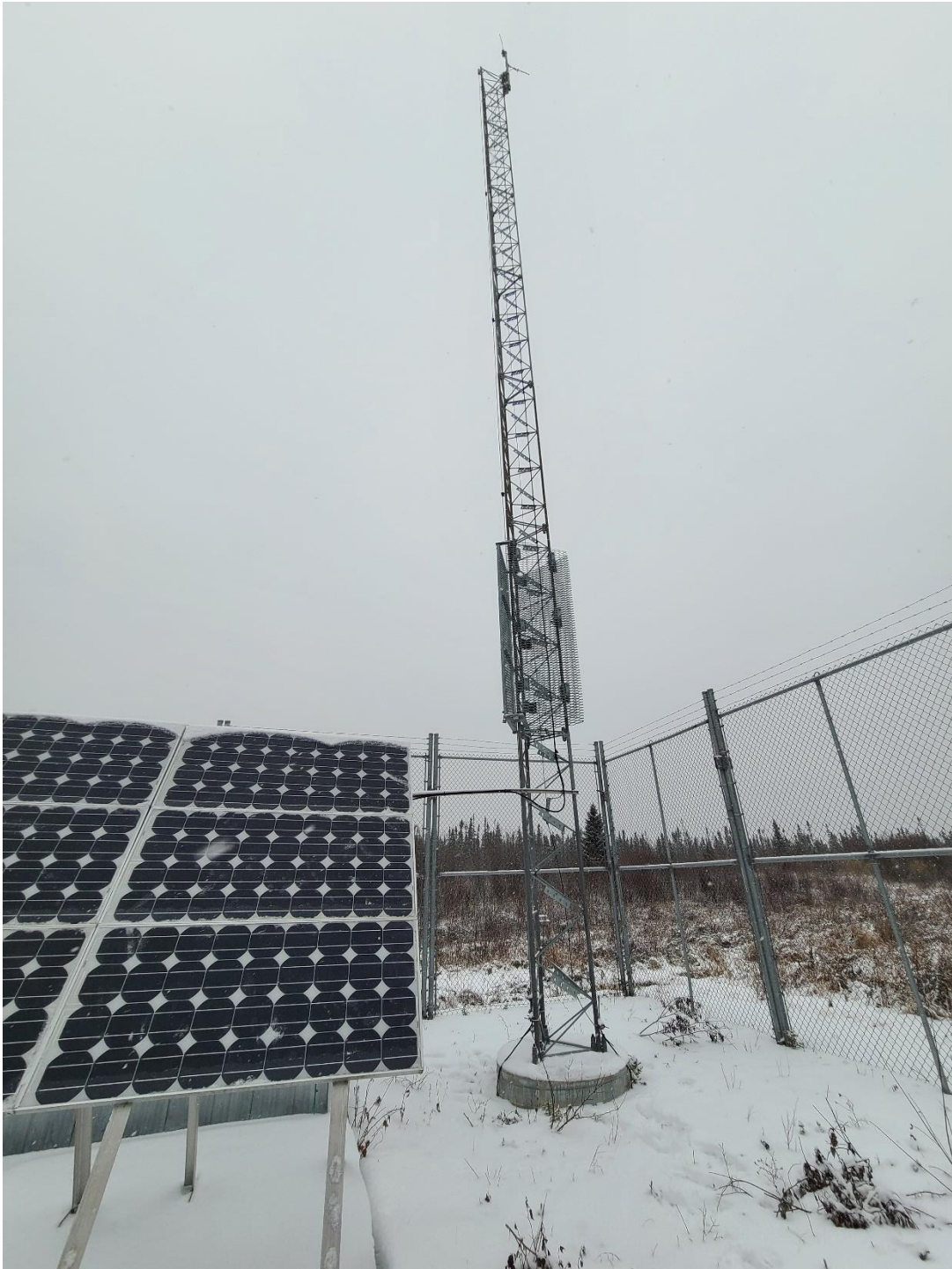
Figure 2: Mile 88.64 Communication Tower
