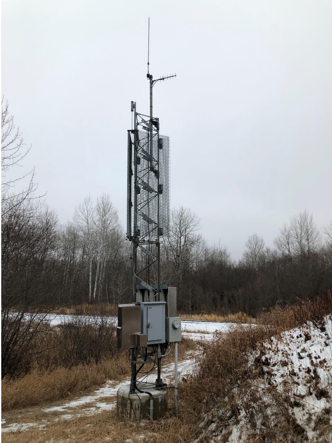
Figure 1: Mile 42.05 Communication Tower
