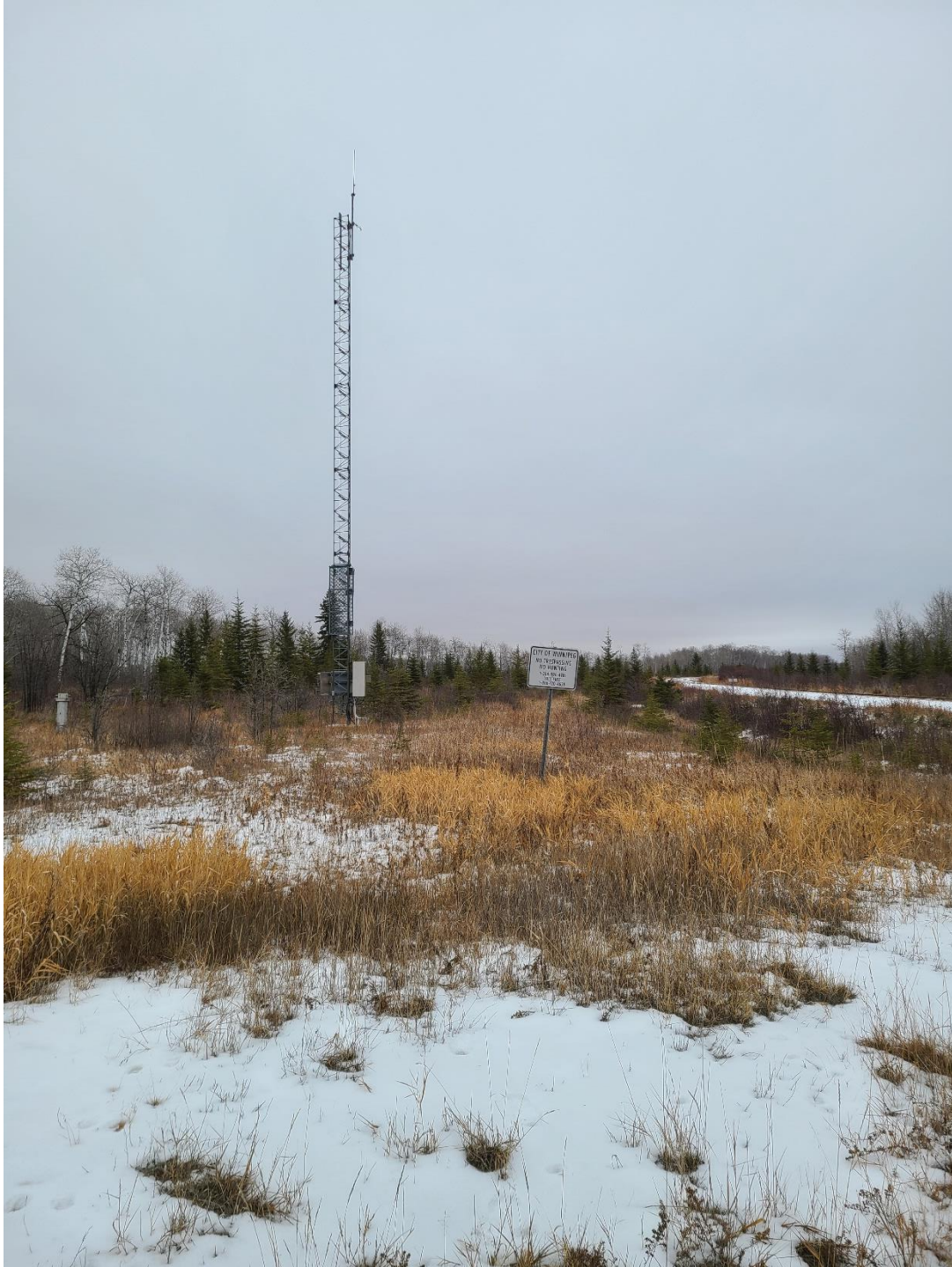
Figure 1: Mile 34.40 Communication Tower
