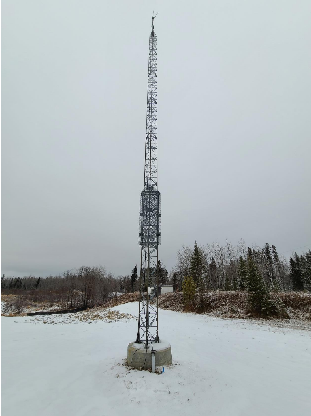
Figure 1: Mile 77.63 Communication Tower
