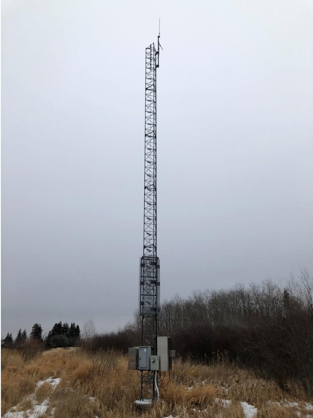
Figure 1: Mile 56.71 Communication Tower
