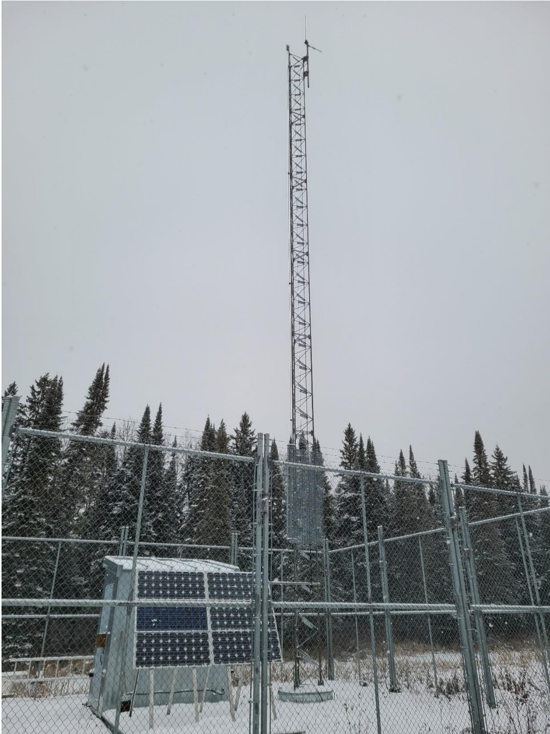
Figure 1: Mile 93.69 Communication Tower
