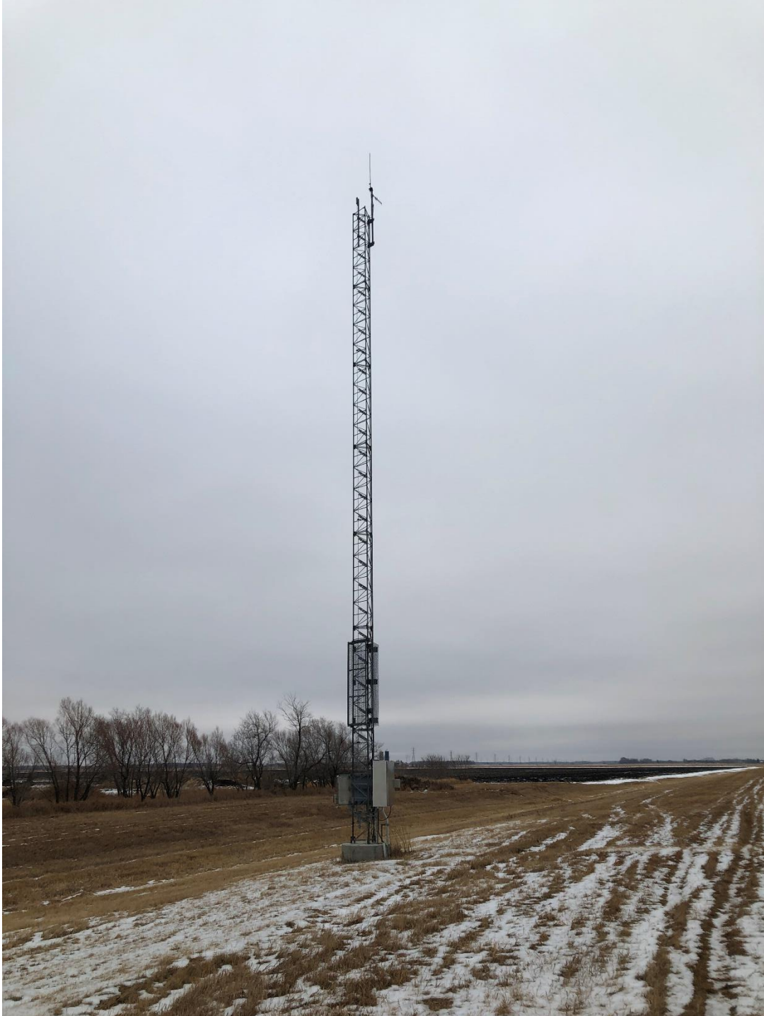
Figure 1: Mile 22.53 Communication Tower
