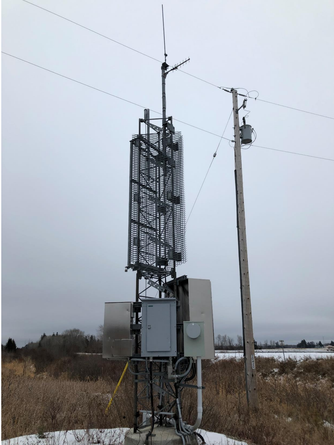
Figure 1: Mile 64.08 Communication Tower
