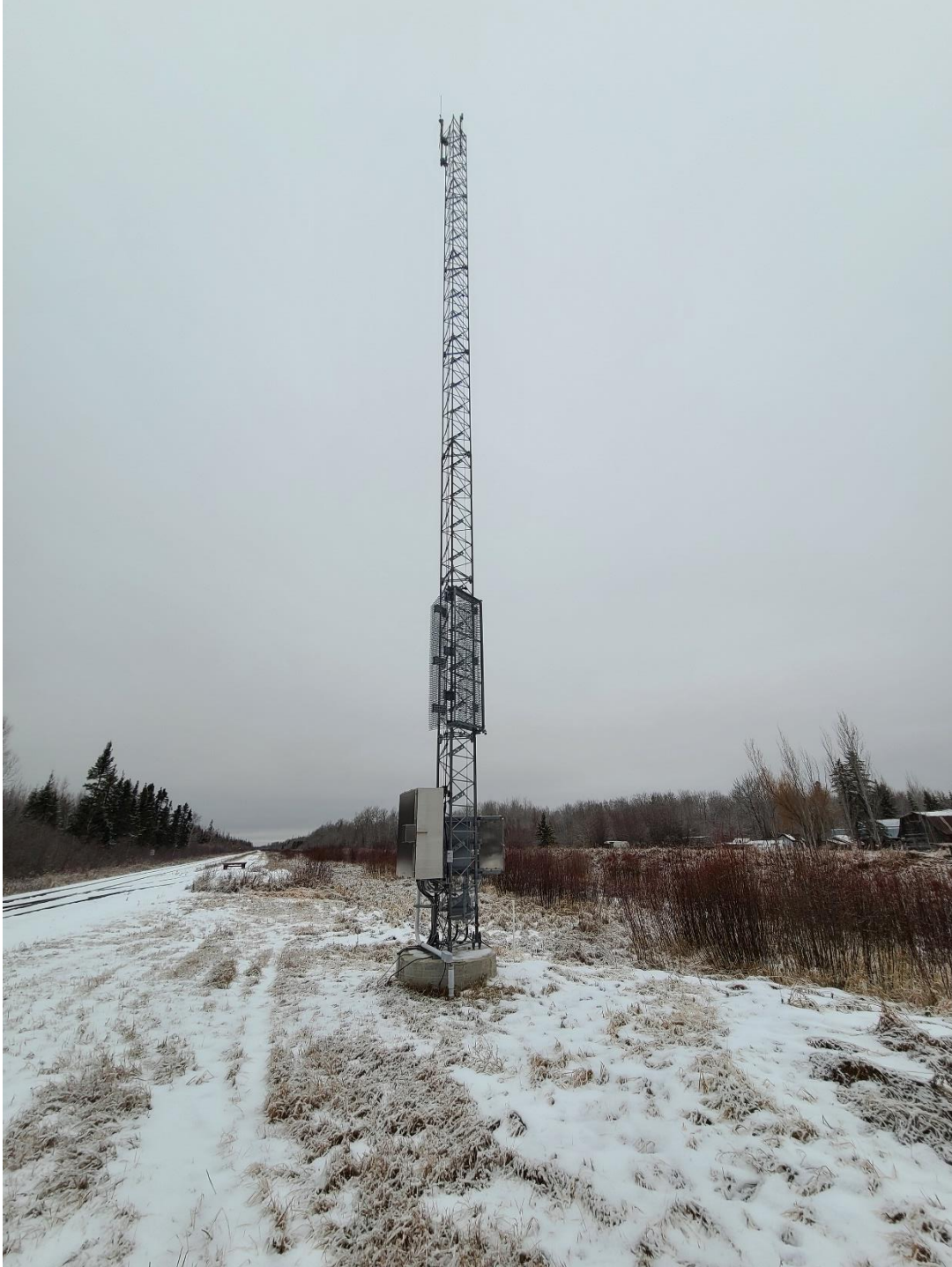
Figure 1: Mile 73.63 Communication Tower
