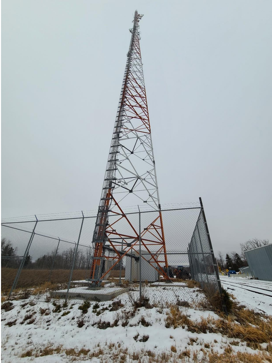
Figure 1: Hadashville Communication Tower
