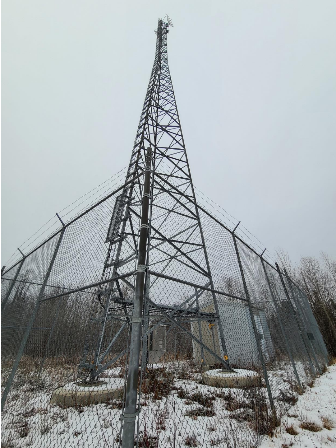
Figure 1: Mile 82.44 Communication Tower
