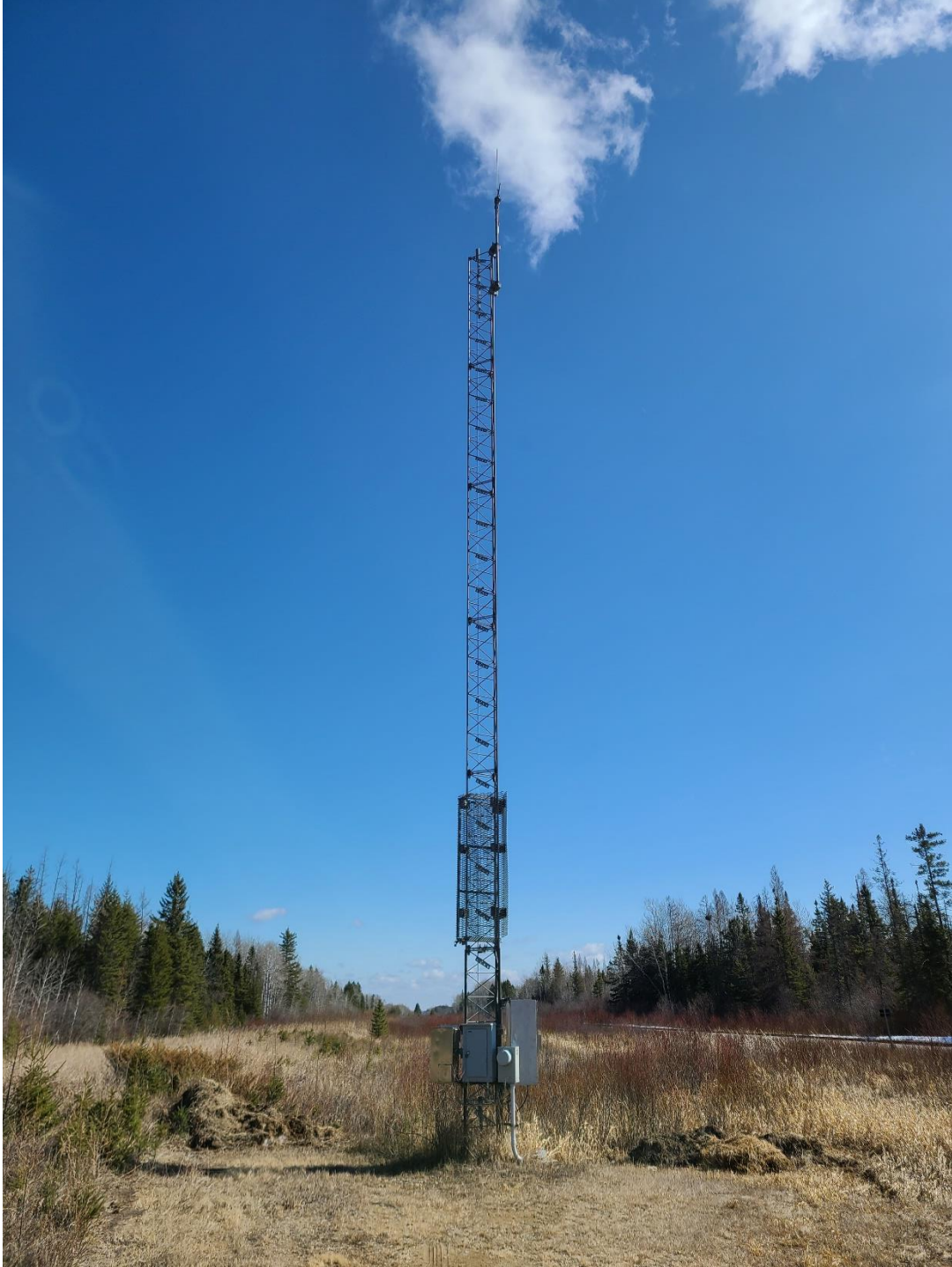
Figure 1: Mile 69.51 Communication Tower
